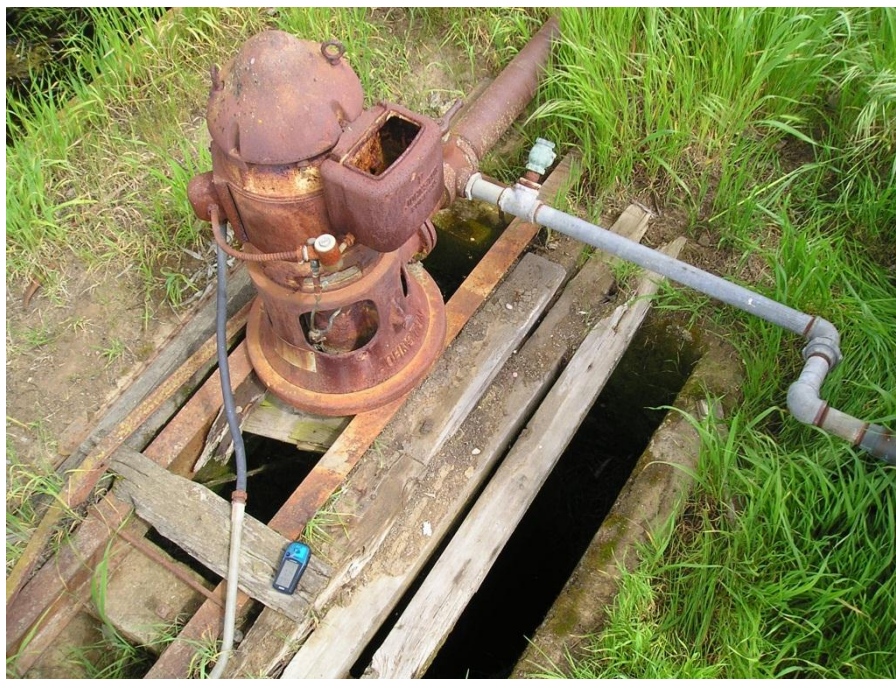
Figure 63. Example of an abandoned well that poses a risk of direct surface runoff spillage into the well casing and into the aquifer (photo courtesy of David Von Aspern and Derek Jacks, Sacramento County).
